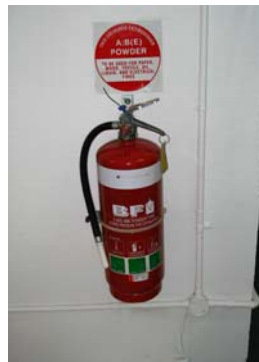
A correctly wall mounted fire extinguisher
